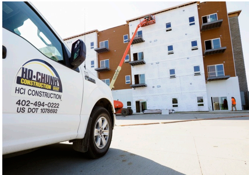
Construction in progress at HCI's Flatwater Crossing master-planned community in South Sioux City, Nebraska.
